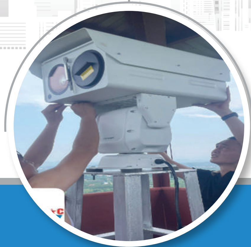
Supply and installation of thermal camera systems for forest fire detection and early warning in Bac Giang and Quang Ninh Provinces
