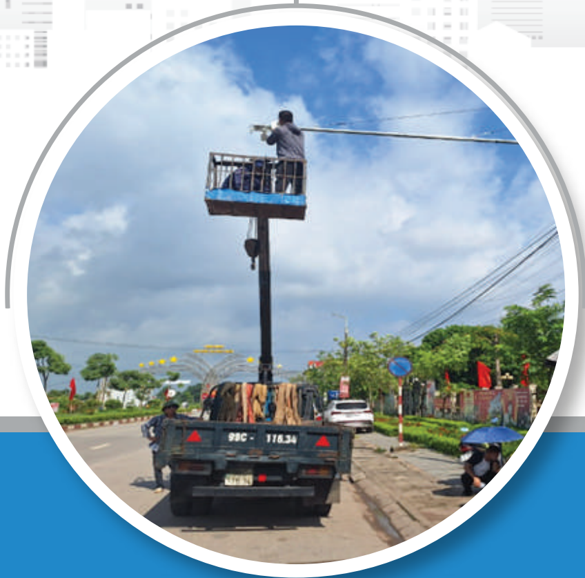
Supply and installation of security surveillance camera system in Lang Giang District, Bac Giang Province
