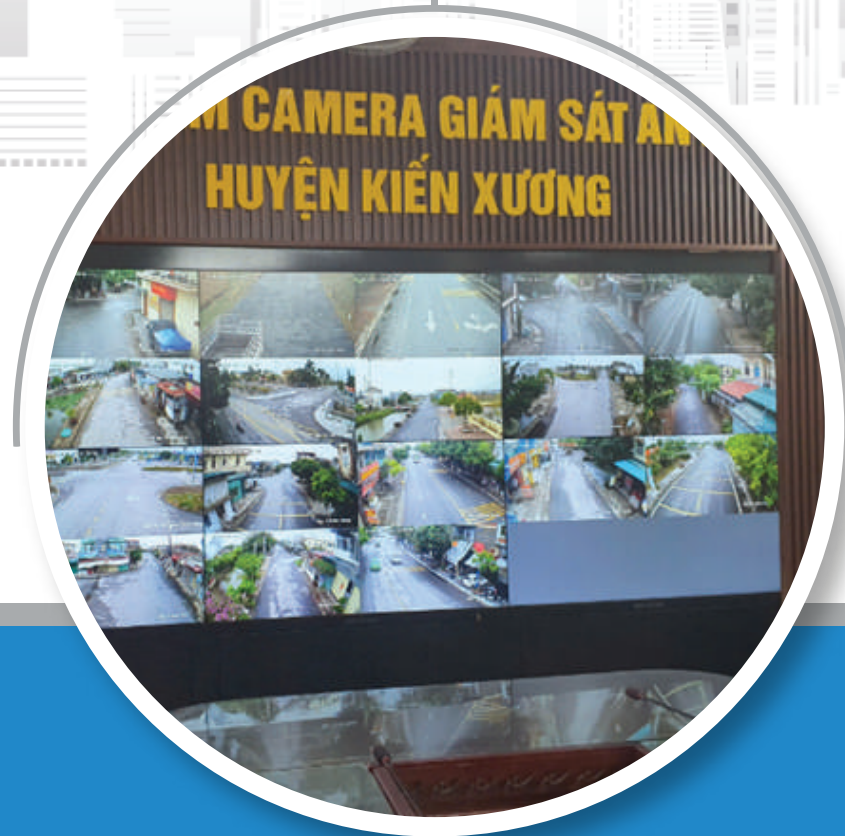
Supply and installation of security surveillance camera system in Kien Xuong District, Thai Binh Province
